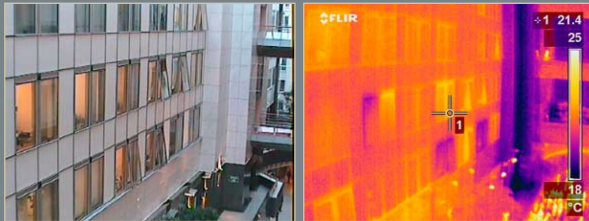
Inside hall - Altiero Spinelli building Loss of heat due to non or badly insulated lift shafts.
